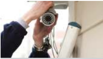
Outdoor Installation Services
