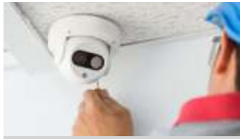
Indoor Installation Services
